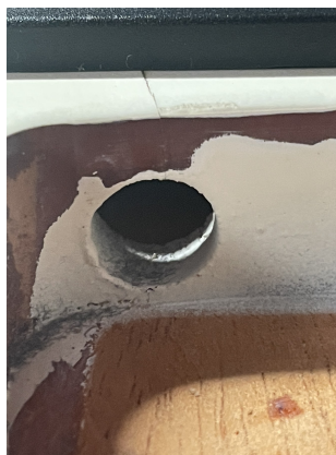
Stress crack / cavity route area before plug repair.
